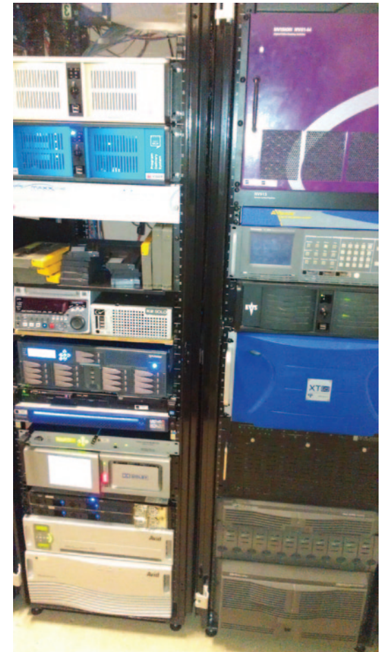
Almost every piece of equipment in these two racks is masquerading as television gear but at their heart they are PCs.
